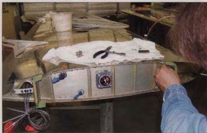
On Day 8 (top), the fiberglass rear door is ready to be test fitted. On Day 9, (above), the final wiring is run through conduit to the wing tips. The inboard fuel tanks, which are separate aluminum vessels, have been plumbed. The Ernsts, intending their Sportsman to be a real utility player, have opted for the direct-reading mechanical fuel gauges.
